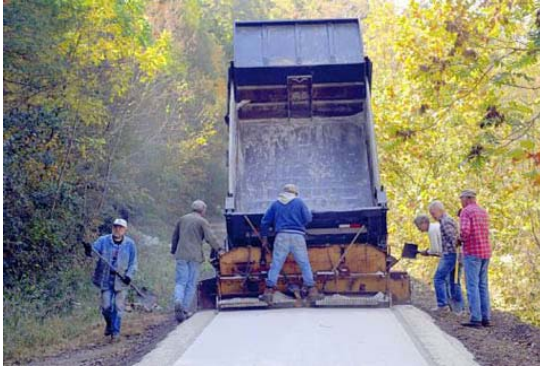
Volunteers apply new trail surface on Montour Trail. Photo courtesy Montour Trail Council
